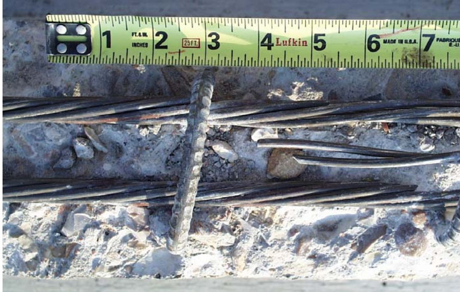
Figure N.18 Photo of Wire Failures in Beam 6 – Location A
