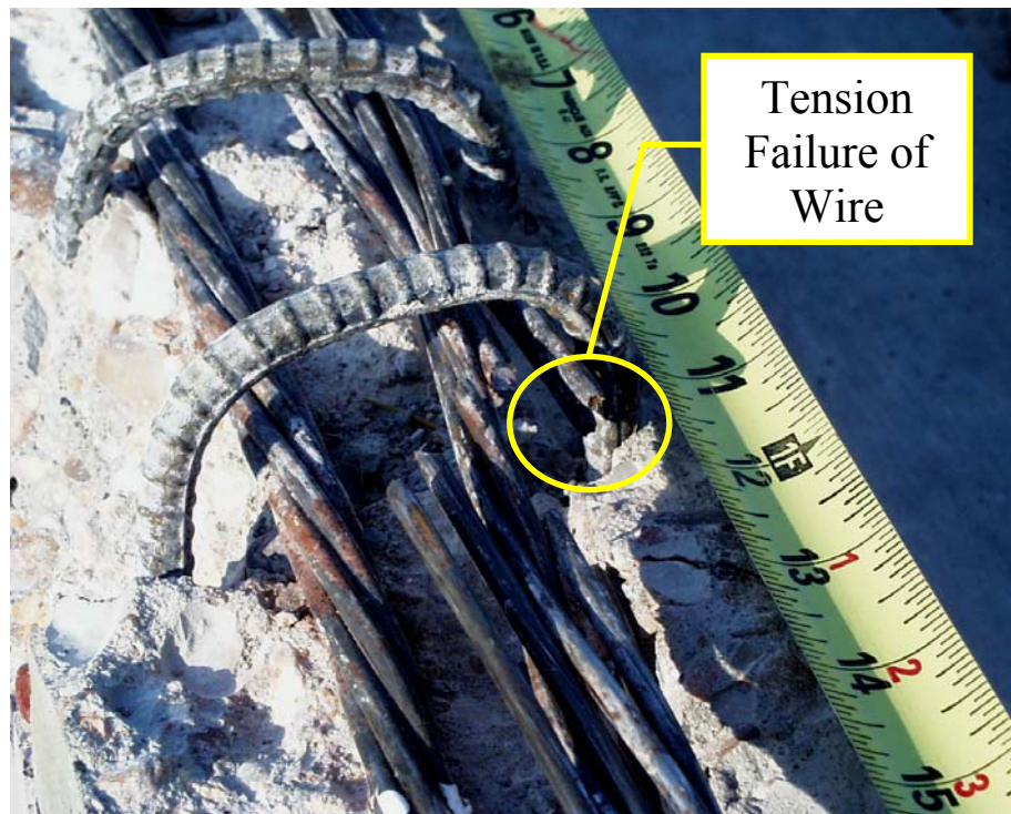
Figure 6.71 Picture of Wire Tension Failure in Beam 6A
