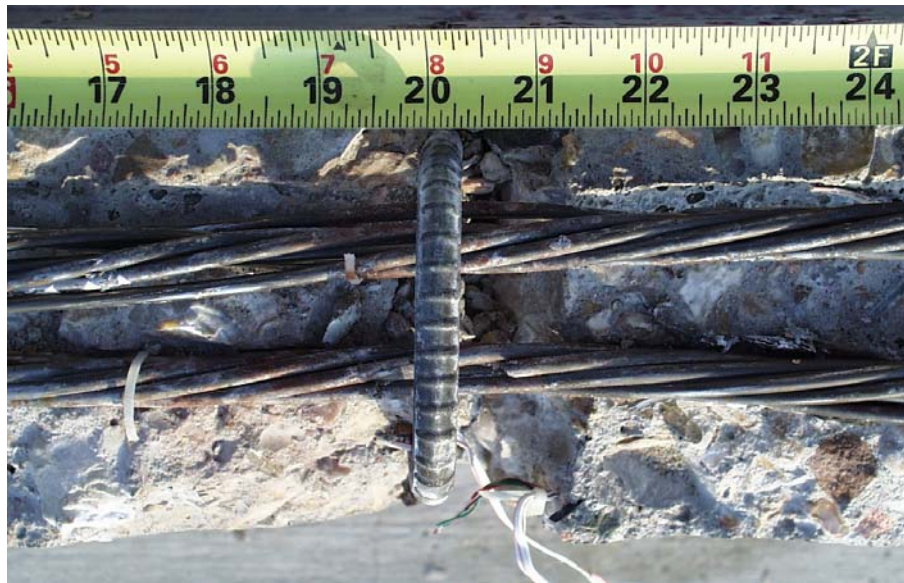
Figure N.20 Photo of Wire Failures in Beam 6 – Location C
