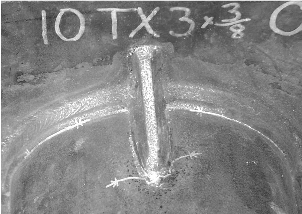
Figure 7.17 Failure of TX 3x3/8 CP Specimen – Note: Paint lines represent extent of visible cracking at termination of stiffener and socket weld toe
