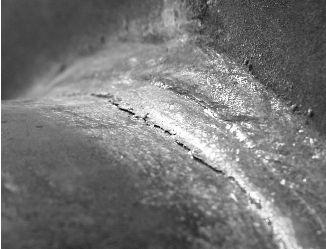
Figure 7.15 Failure of UIT Treated Socket Connection Specimen
