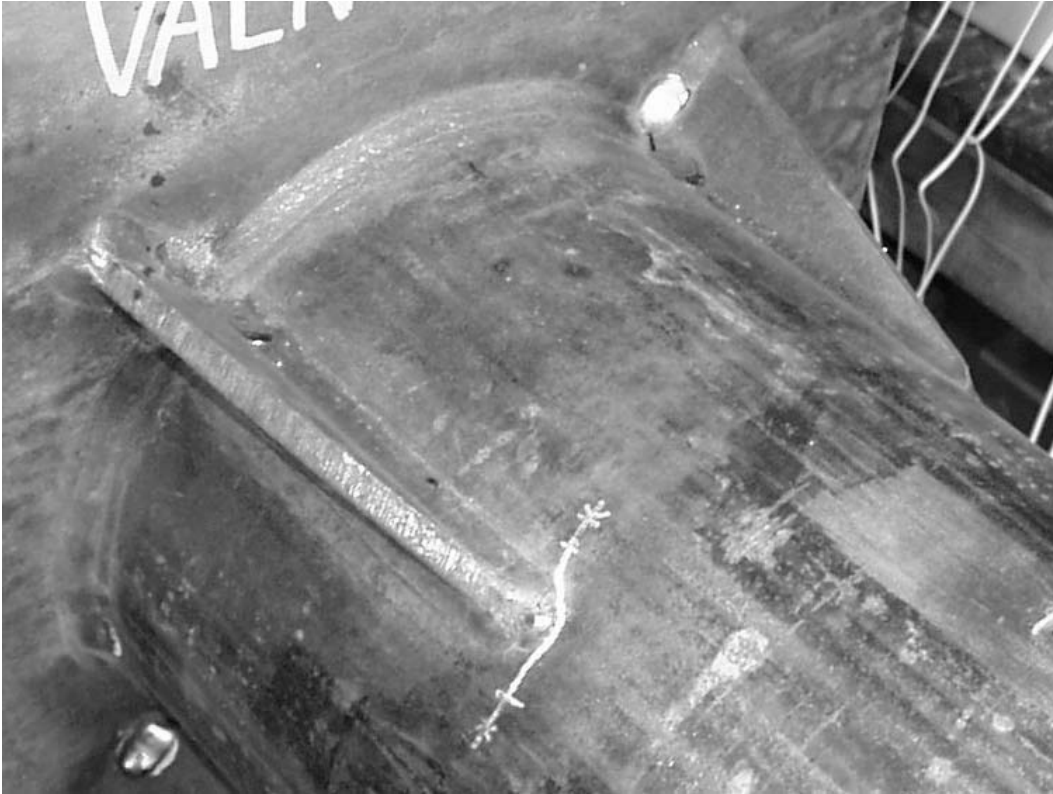
Figure 7.11 Failure of VALN 6x3/8@45 Specimen – Painted line indicates extent of visible cracking, specimen tested at 6 ksi stress range
