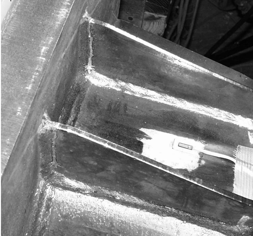
Figure 7.24 Failure of U-Rib Stiffened Specimen – Note: Painted lines represent extent of visible cracking
