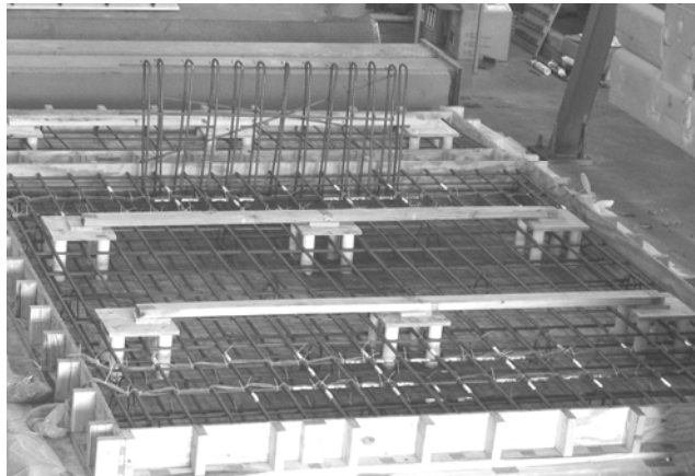
Figure 3.2- Reinforcement layout of the T203 bridge deck and cast-in-place barrier test specimens
