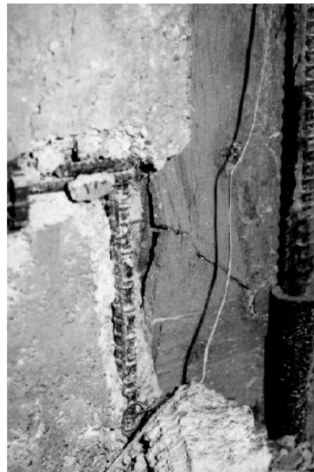
Figure 4.5: Crushing at Toe of Wall
