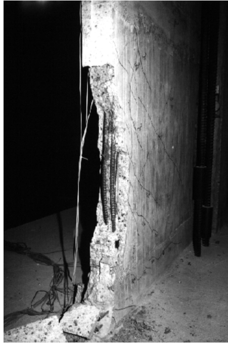
Figure 4.11: Buckled Reinforcement in Closure Strip
