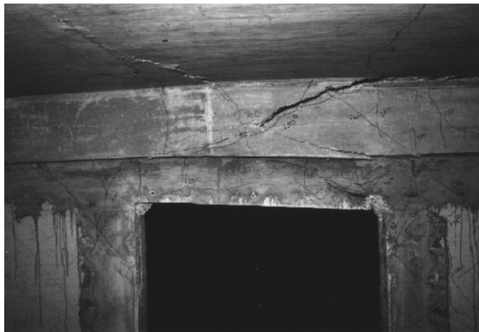
Figure 4.13: Failed Coupling Beam During East Direction Loading
