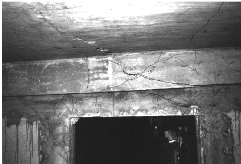
Figure 4.10: Failed Coupling Beam During West Direction Loading
