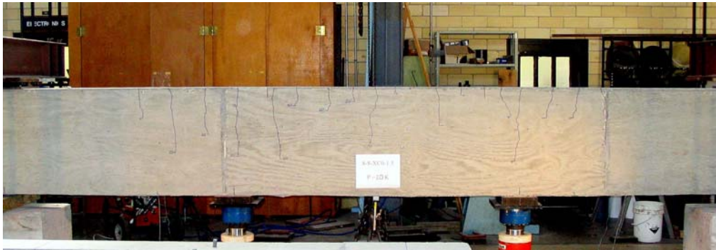
Figure 5-13: Cracking of typical unconfined specimen at early loading stages
