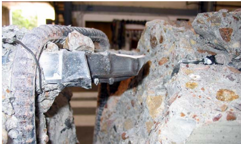
Figure 5-31: Ruptured #8 bar in specimen 8-5-OC2-1.5
