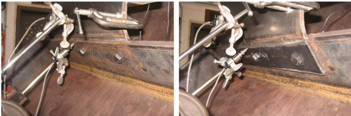
Figure 5.16 Bolted Bent Plate Connection on (a) Prying Side and (b) Restricted Side
