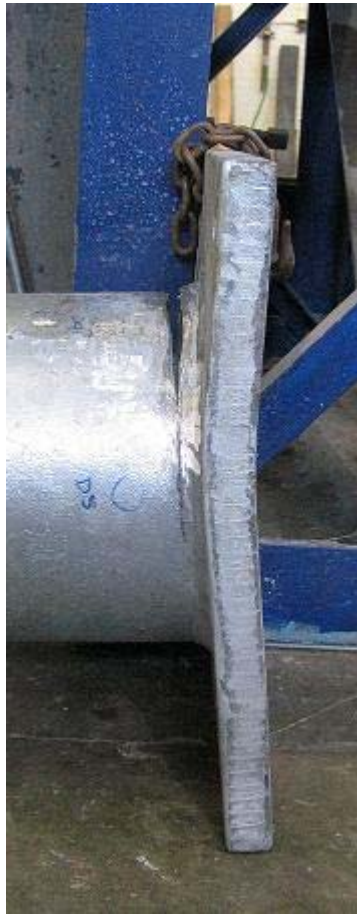
Figure 4.4.2 Side View of Mast Arm TXuDLGP After Cracking
