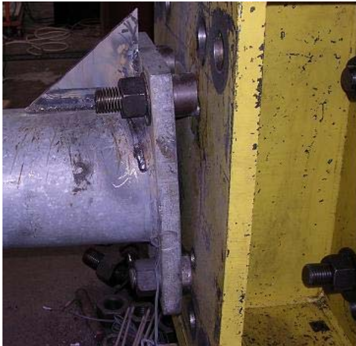
Figure 7.3.1 Beveled Washers Connecting the Mast Arm Baseplate to the Load Box
