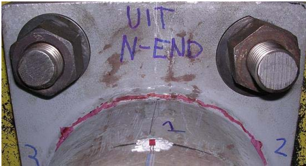
Figure 8.3.2 Highlighted Fatigue Crack on Specimen DU Mast Arm Weld Toe Along the UIT Application Line (90,680 cycles)
