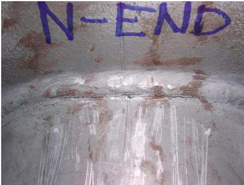
Figure 8.3.1 Close-up of Fatigue Crack on Specimen DU Mast Arm Weld Toe Along the UIT Application Line (90,680 cycles)
