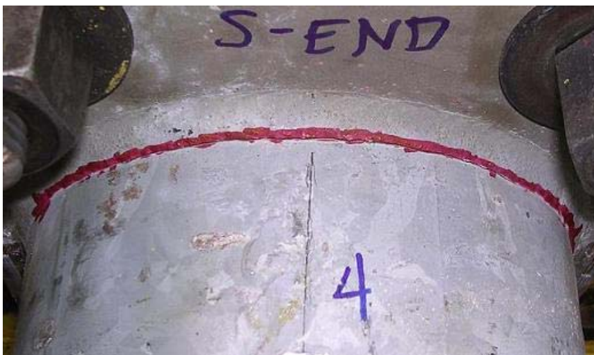
Figure 8.3.6 Highlighted Fatigue Crack Along Mast Arm Weld Toe of Specimen DN (224,905 cycles)
