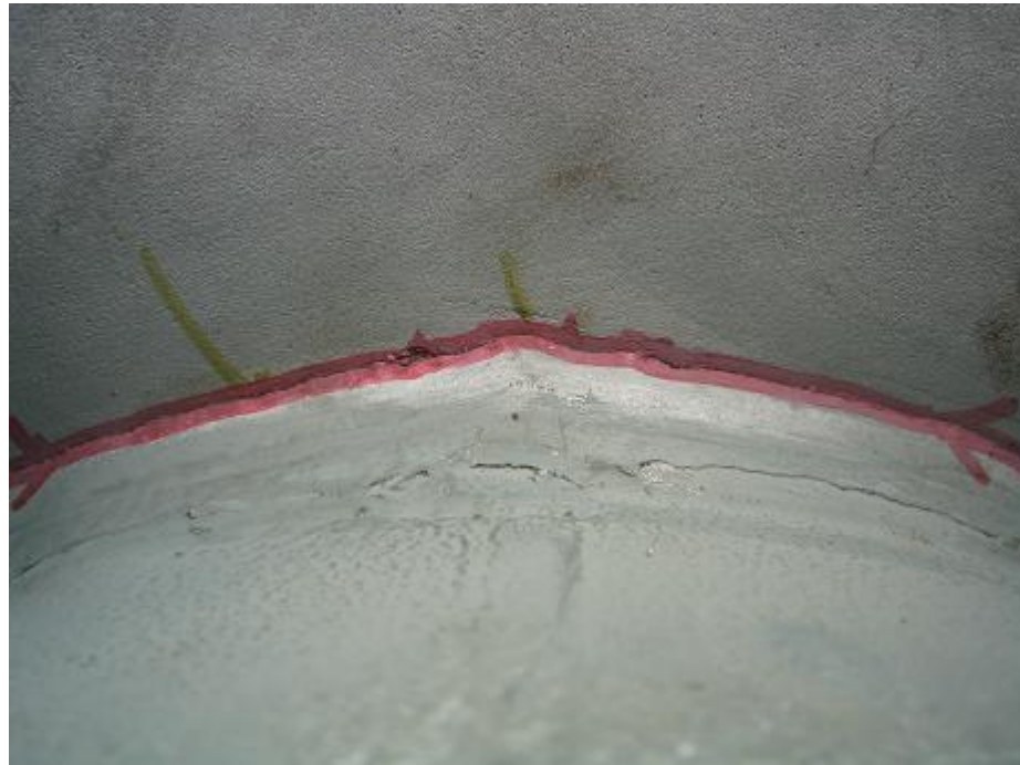
Figure 3.1.1 Fatigue Crack Along Un-Treated Base Plate Weld Toe [29]
