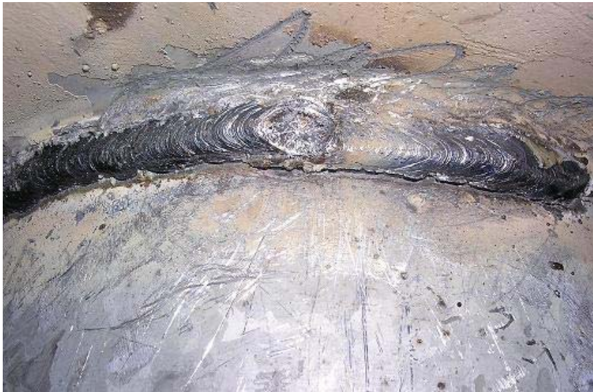
Figure 8.3.3 Close-up of Fatigue Crack on Specimen DU Mast Arm Weld Toe Along the Weld Repair (116,876 cycles)
