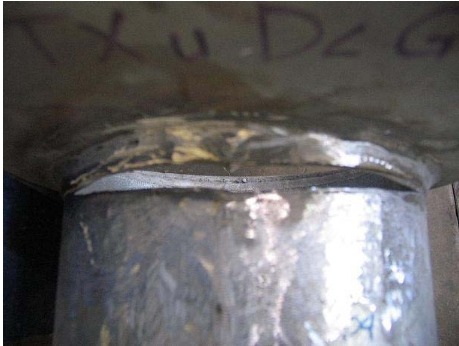
Figure 4.4.1 Top View of Crack Along the Mast Arm Weld Toe of TXuDLGP
