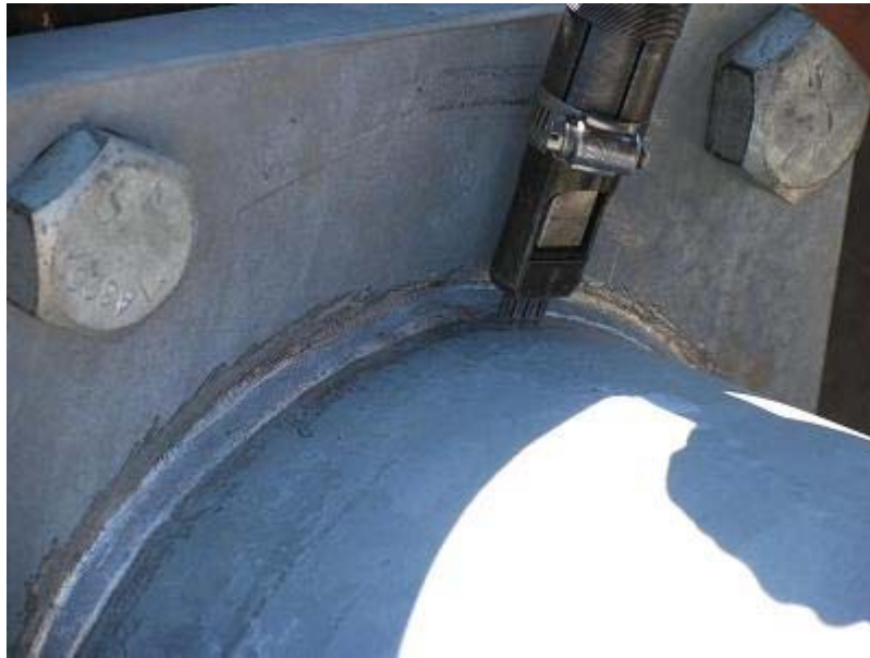
Figure 5.4.2 Employee’s First UIT Application to a Mast Arm Weld
