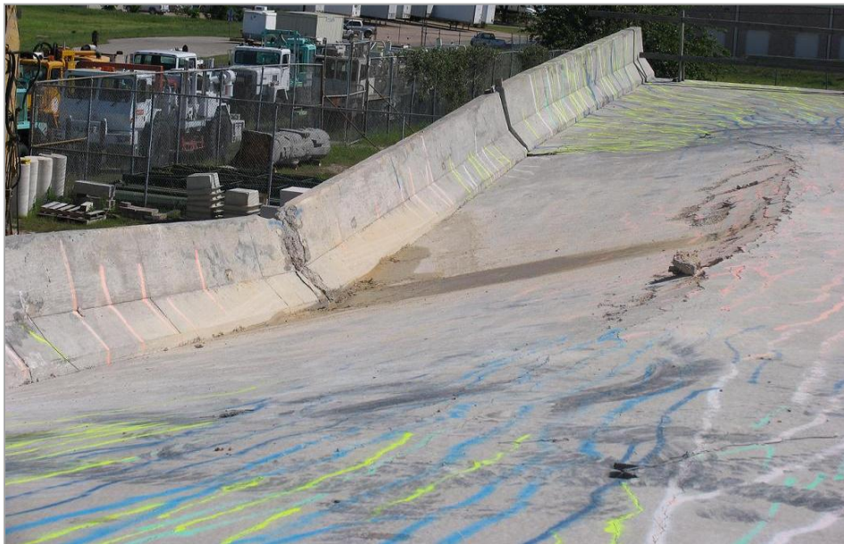
Figure 5-1: Overall view of the damaged deck
