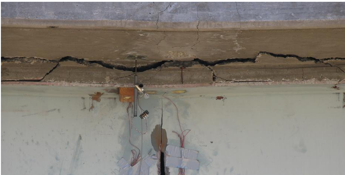
Figure 4-5: Localized shear stud failure
