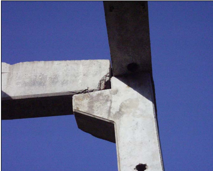
Figure 2.9 Concrete Spalling due to Impact when the Column Rotates
