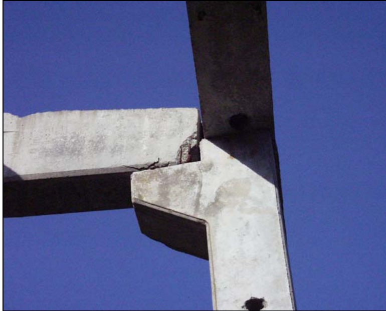
Figure 5.1 Concrete's Spalling off Due to Impact when Column Rotates
