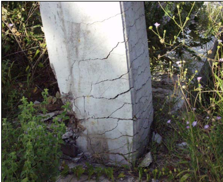
Figure 2.6 Plastic Hinge at the Base of Columns in a One-story Building near Adapazari
