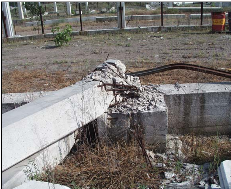
Figure 2.7 Plastic Hinge at the Base of Columns in a One-story Building near Gölcük
