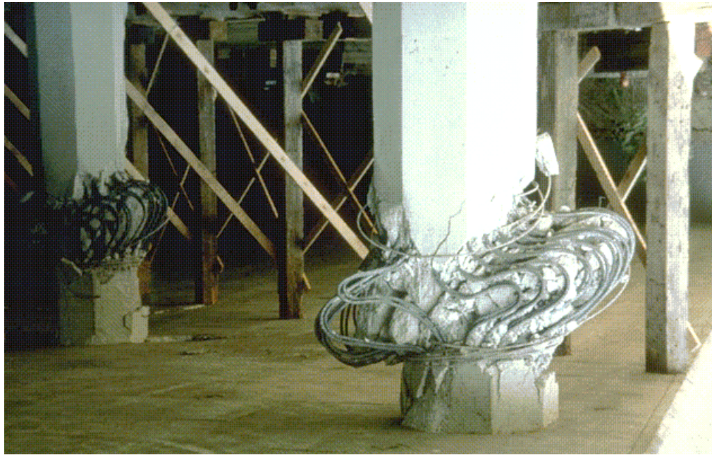
Figure 1.1 Buckling of freeway support column's reinforcement under the Simi Valley Freeway at the north end of the San Fernando Valley during the Northridge earthquake in California 1994 (photo: Ta-Liang Teng), from: http://www.scecdc.scec.org/slidesho.html
