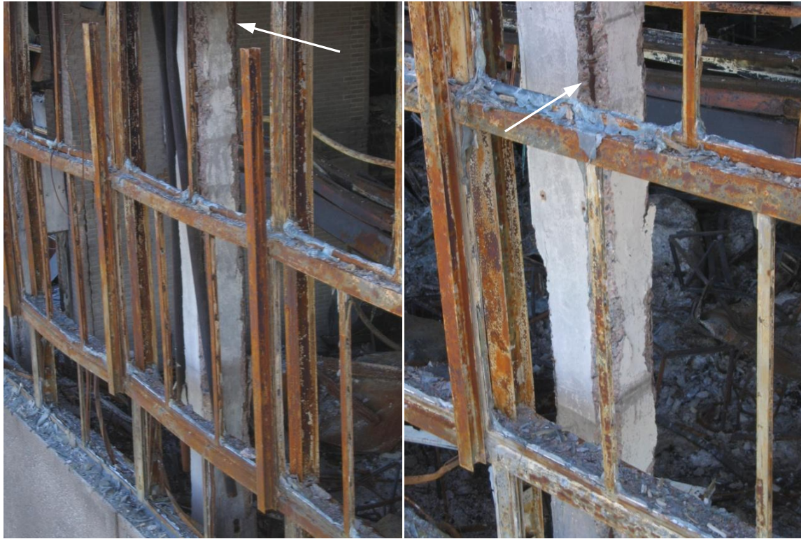
Figure 3.5 Exterior Columns After the Fire with Spalled Concrete Cover
