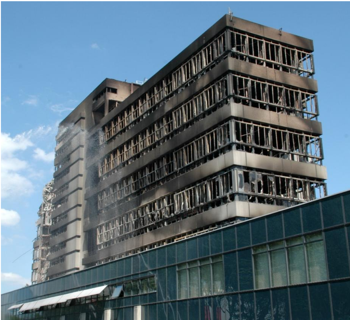
Figure 3.8 North-East Wing After the Fire (©Rob Jastrebski)
