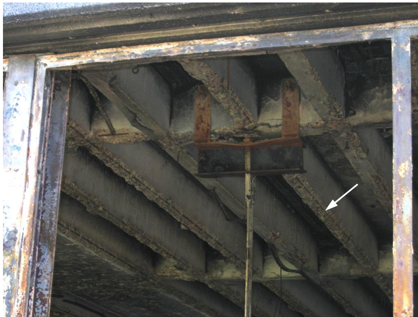
Figure 3.6 Floor Joist After the Fire with Spalled Concrete Cover
