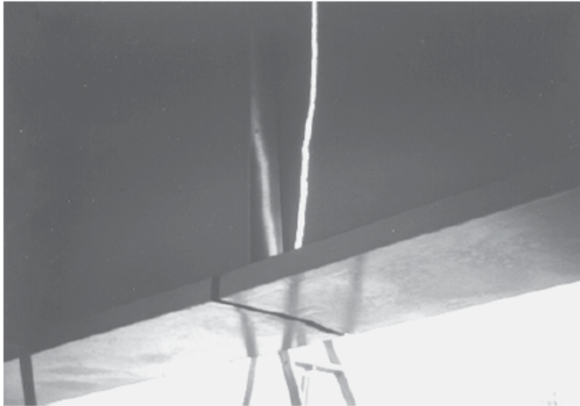
Figure 1.2: Fracture in Exterior Girder of Neville Island Bridge, 1977 (Conner, Dexter, and Mahmoud, 2005)
