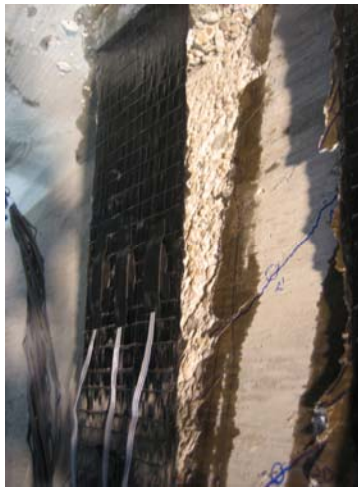
Figure 2-12 An experimentally debonded CFRP strip
