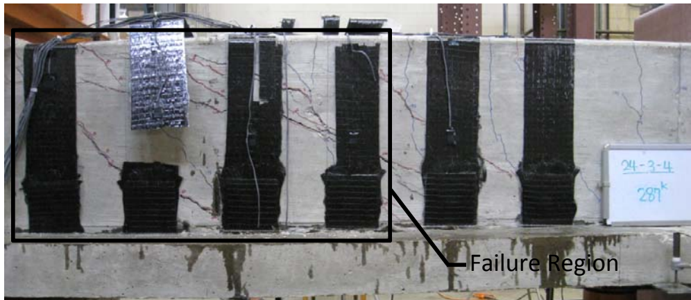
Figure 4-49 Failure region of 24-3-4 (east)
