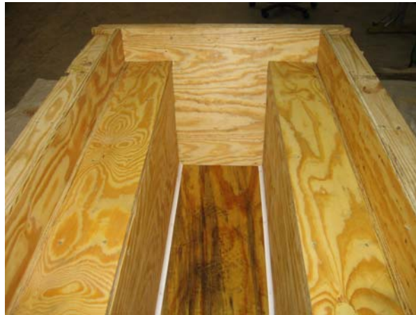
Figure 3-6 Chamfer strips provided at 90 degree corners to provide a sufficiently rounded corner for CFRP materials
