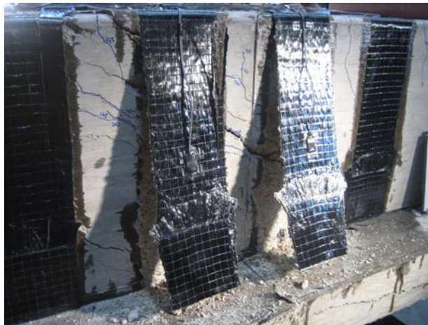
Figure 4-77 CFRP anchorage failure observed during 24-2.1-1
