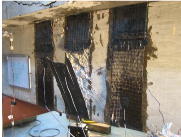
Figure 2-13 Rupture of a CFRP strip
