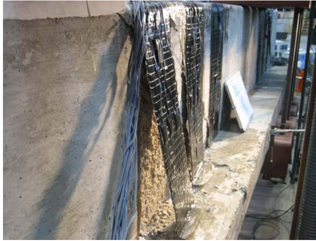
Figure 4-107 Debonding of CFRP strips during 24-1.5-2
