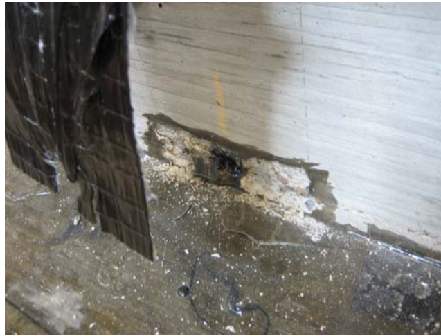
Figure 5-6 Premature CFRP anchor failure (24-3-3)
