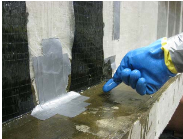
Figure 5-4 Large gaps between the CFRP and concrete during CFRP installation of 24-3-3
