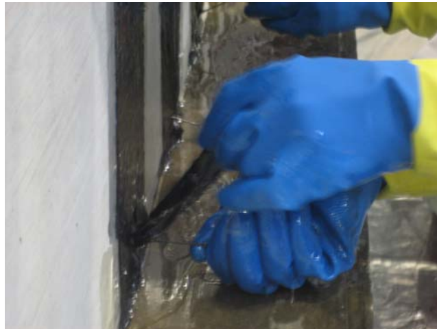
Figure 2-43 Using a rebar tie to properly insert the CFRP anchor into a predrilled hole.
