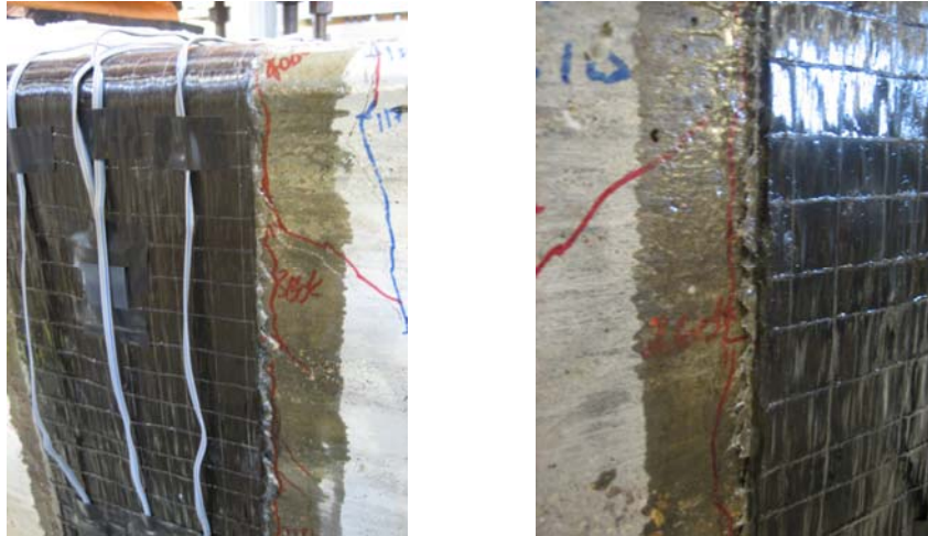
Figure 4-97 Observed debonding during test 24-1.5-1R
