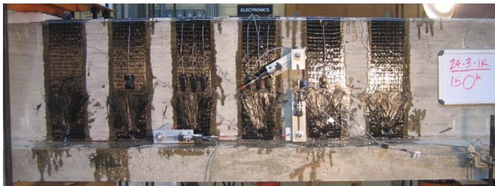
Figure 4-11 24-3-1R at 150-kips applied load (79-kips applied shear)
