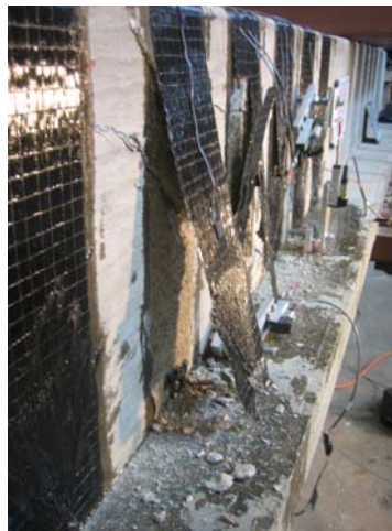
Figure 4-8 CFRP anchor failure observed during 24-3-1R
