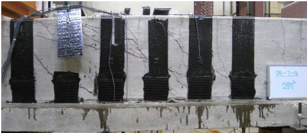
Figure 5-14 CFRP rupture failure observed during 24-3-4
