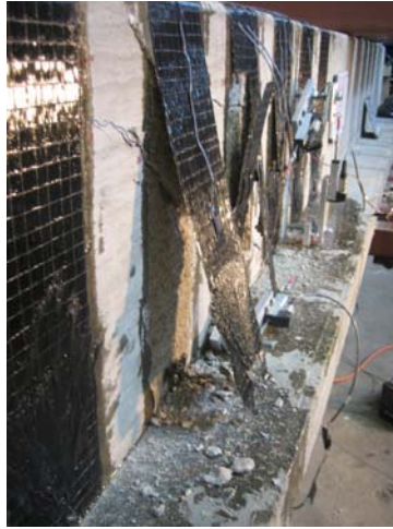
Figure 3-40 Rupture of the CFRP anchor near the anchor hole opening
