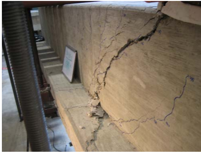
Figure 4-112 Failure observed during 24-1.5-3
