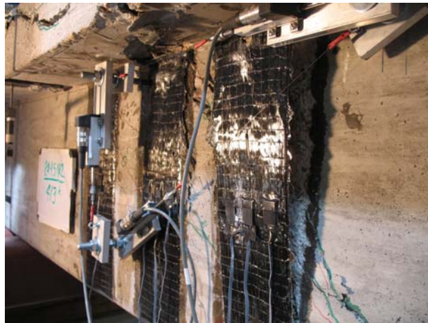
Figure 4-101 Anchorage failure of 24-1.5-1R2 (west side)
