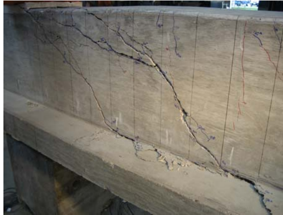
Figure 4-19 Large cracking observed during 24-3-2
