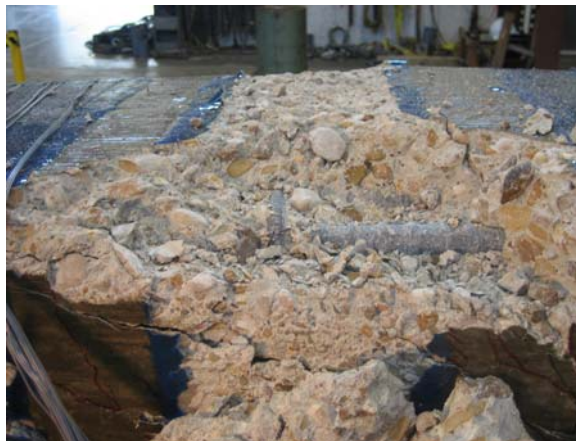
Figure 4-66 Removed concrete cover, test 24-3-6
