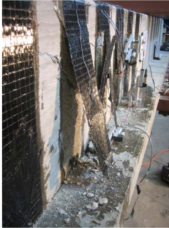
Figure 5-11 Anchor rupture associated with 24-3-1R
