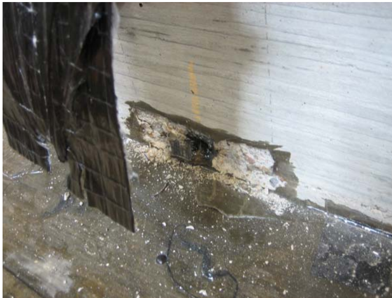
Figure 5-12 Anchor rupture associated with 24-3-3
