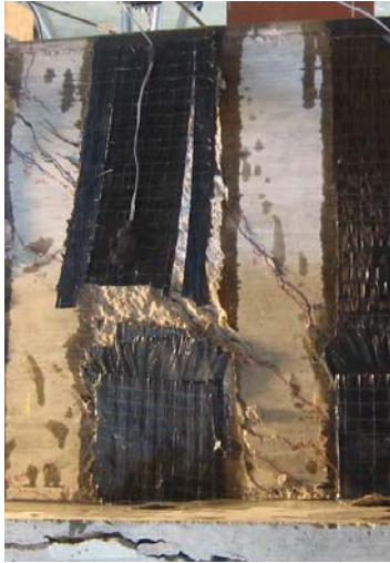
Figure 3-44 Failure of CFRP strip with new anchorage detail installed
