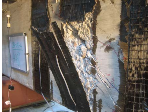
Figure 4-117 Rupture of a CFRP strip during 24-1.5-4
