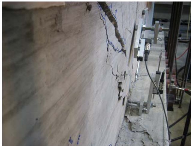
Figure 4-111 Bulging of concrete observed during 24-1.5-3 (west)
