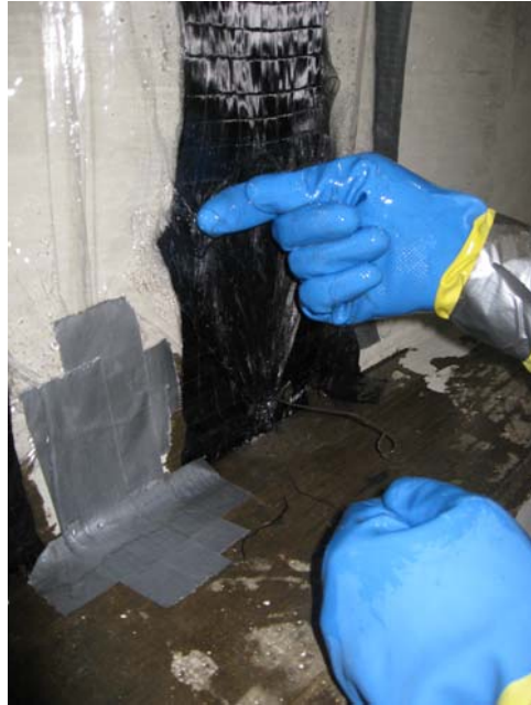
Figure 5-5 Gaps observed near the edges of the CFRP strips (24-3-3)
