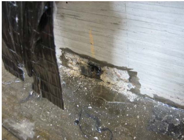
Figure 4-30 Premature CFRP anchor rupture, test 24-3-3
