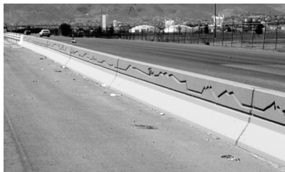
Figure 3.17: Colored and Textured Traffic Barrier in Same Area Is Free of Graffiti
