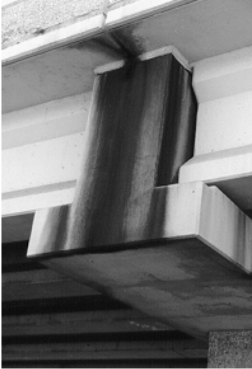
Figure 3.15: Staining Due to Runoff from Superstructure
