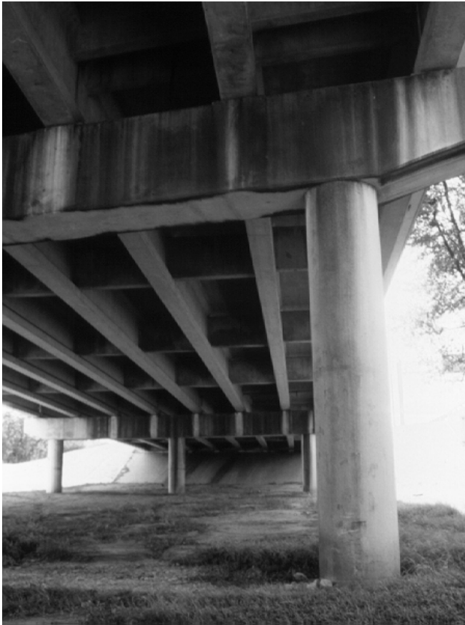
Figure 1.4: Staining of Substructure
