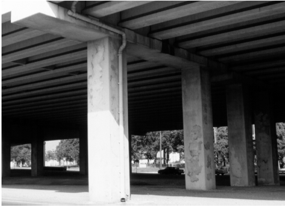
Figure 1.6: Columns in Need of Repainting
