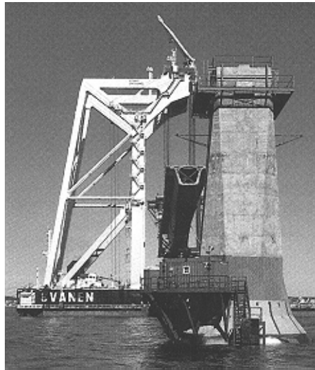
Figure 2.44: Template in Place atop Pier — Svanen with Girder in Background (from Ref. 21)
