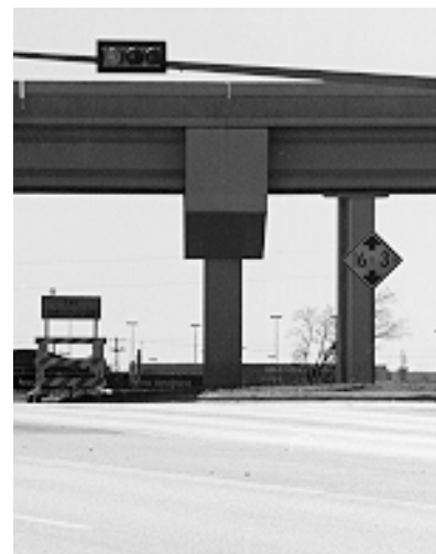
Figure 3.5: Pier Appears Inadequate beneath Large Cap
