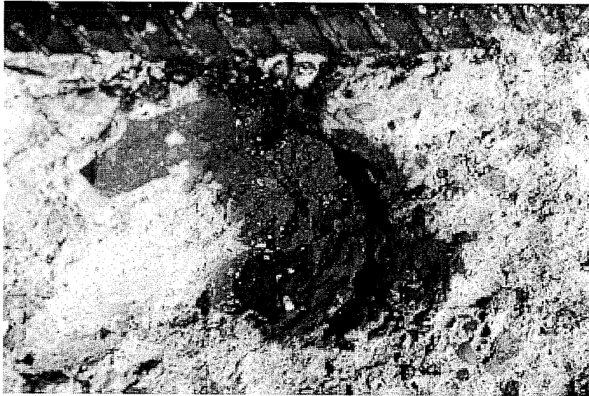
Figure 5.8 Green Corrosion Fluid on Beam 34.
