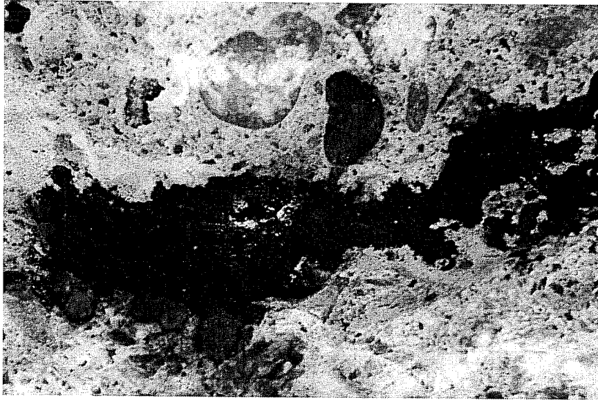
Figure 5.33 Active Corrosion on Concrete Bent Black Bar Side (1B8).
