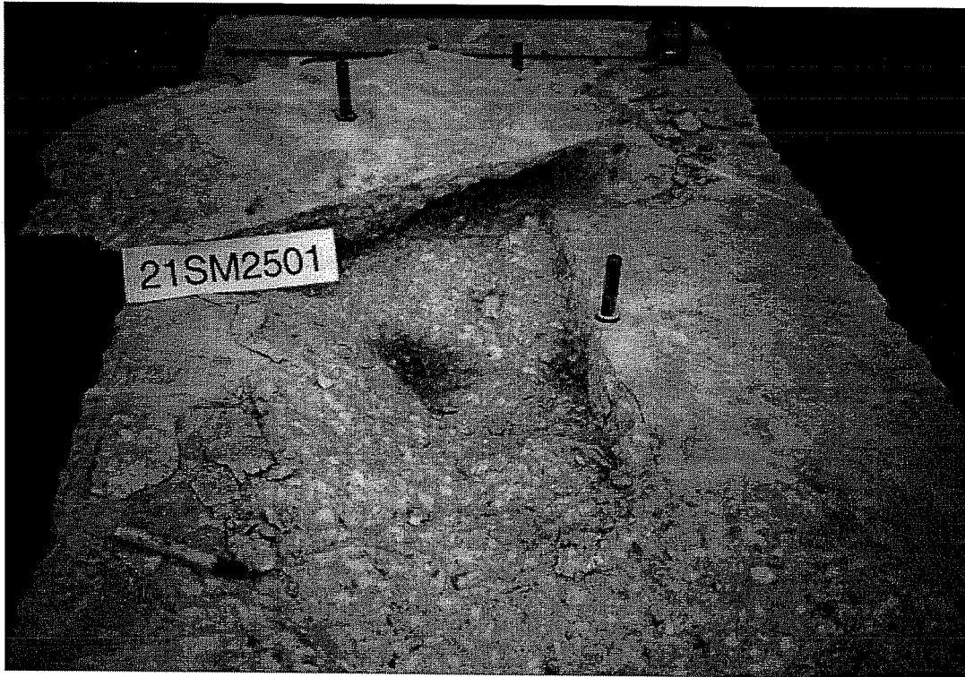
Failure Picture of Test 21SM2501, Spacing of 2.5 * h_{ef} , UC1, Static, Concrete Breakout at Anchor
