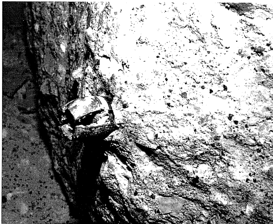
Failure Picture of Test 23M34T4, UC1 3/8", Pure Tension, Details of Expansion Elements
