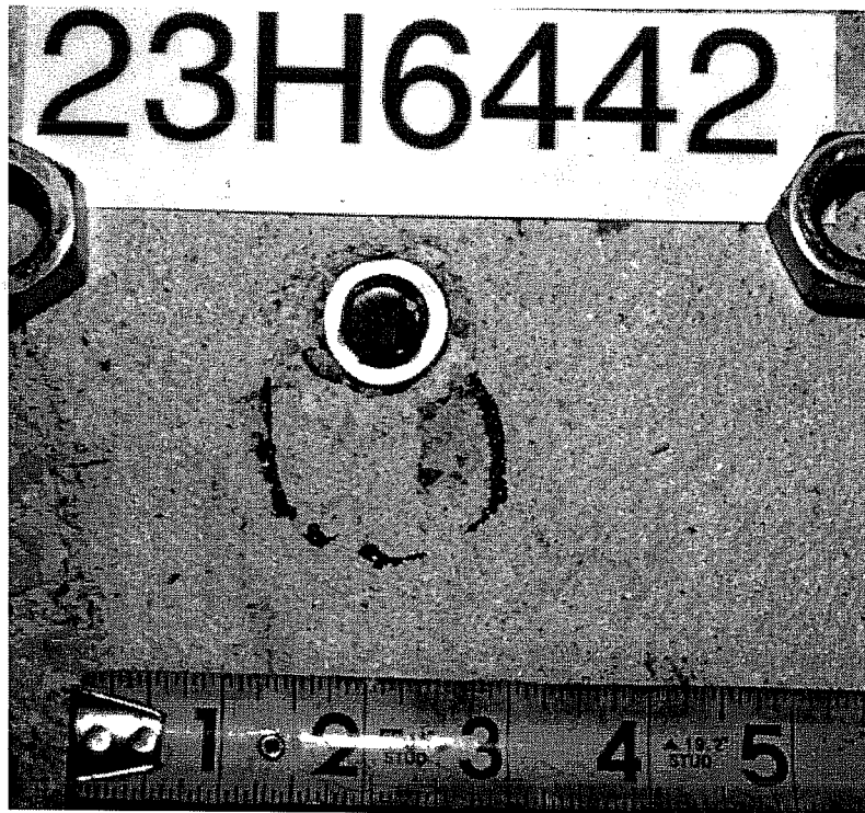
Failure Picture of Test 23H6442, Sleeve M16, Oblique Tension 45°
