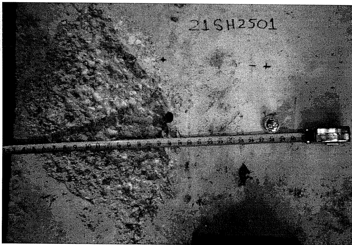
Failure Picture of Test 21SH2501, Spacing of 2.5 * h_{ef} , Sleeve, Static, Concrete Failure at Anchor
