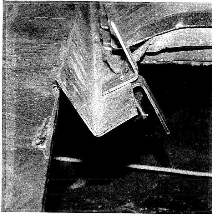
Figure 4.17 Support angle warping at tension corner.
