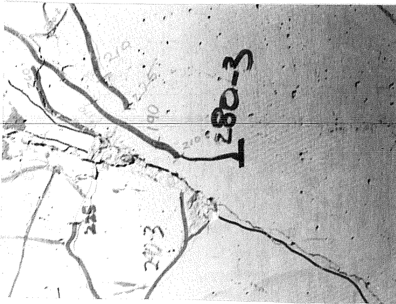
Fig. 3.12 Large flexural crack with some concrete spalling at 0.5% drift. Interior of first level beam, north of south pier
