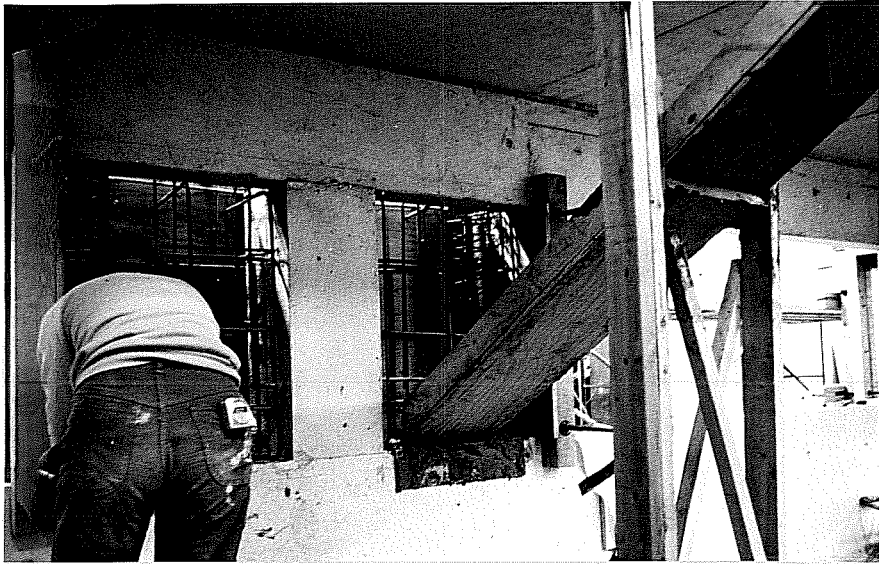
Fig. 2.32 Concrete was placed from the interior of the frame using a chute which emptied into the formwork.
