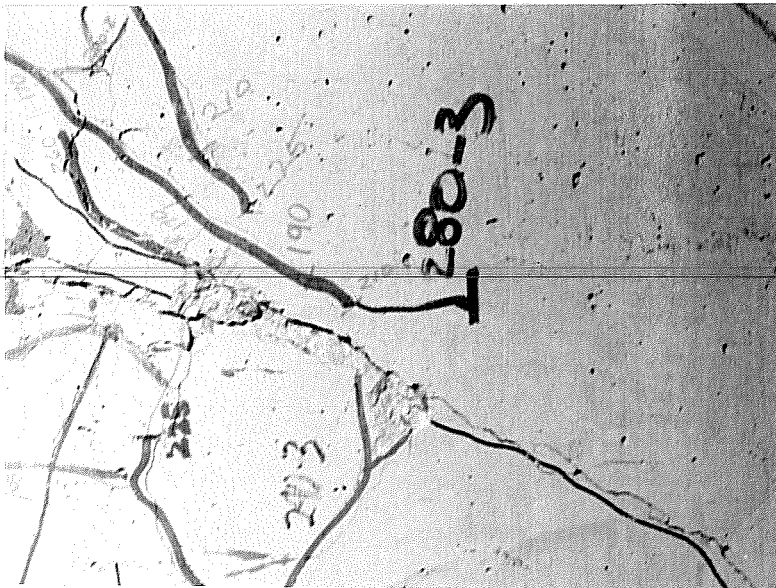
Fig. 3.12 Large flexural crack with some concrete spalling at 0.5% drift. Interior of first level beam, north of south pier.
