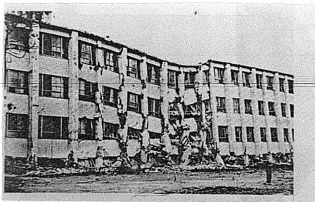
Fig. 1.3 Severe damage due to short column shear failure. Hokodate College, Tokachi-oki 1968 [10]
