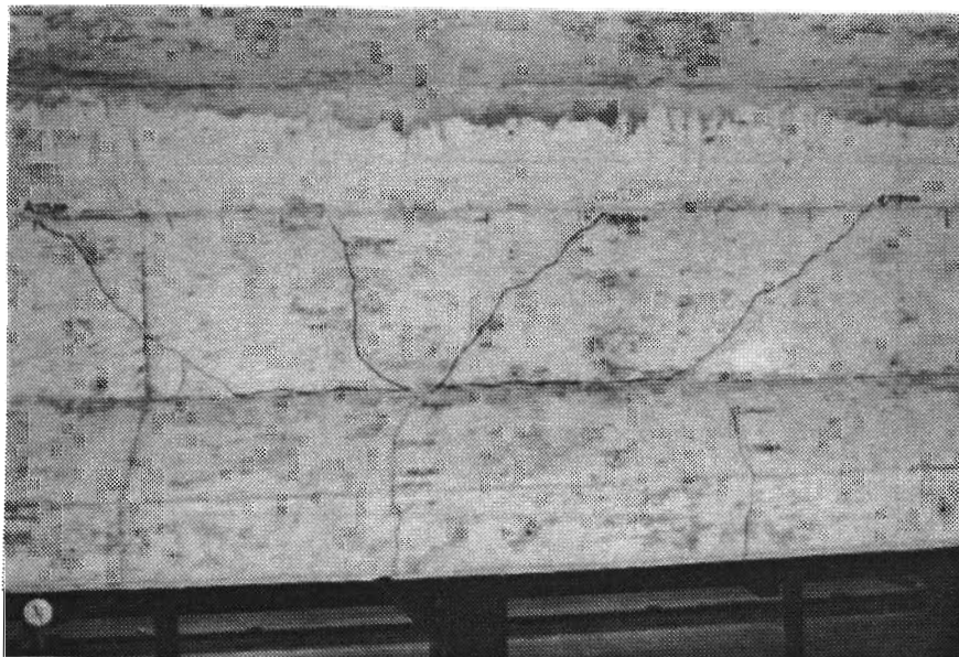
Fig. 4.38 East side (top) and west side (bottom) torsional cracking observed in the flexural failure zone
