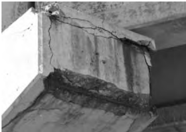
Figure 1.2 Damage at downstream endcap
