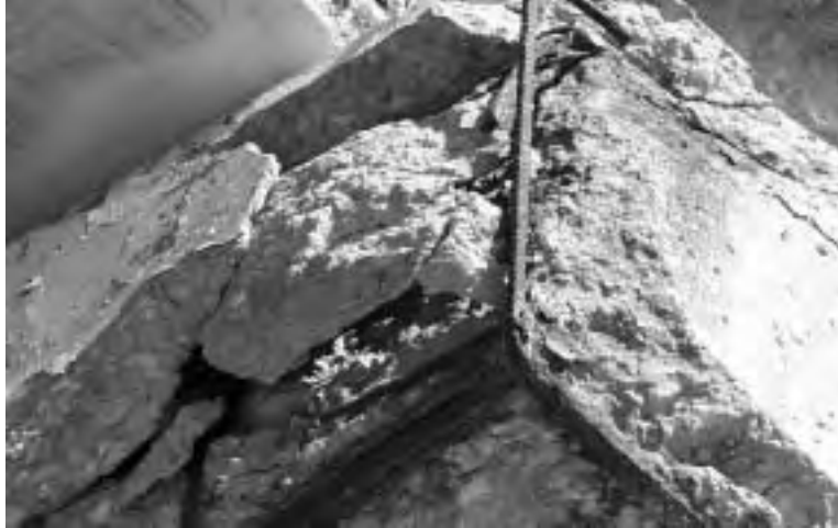
Figure 5.2 Closeup of corrosion damage on Structure #8
