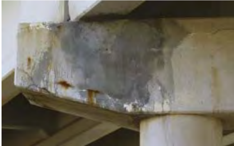
Figure 5.15 Delaminations and corrosion stains on a downstream endcap
