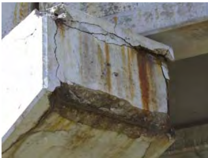
Figure 5.1 Endcap damage to Structure #5
