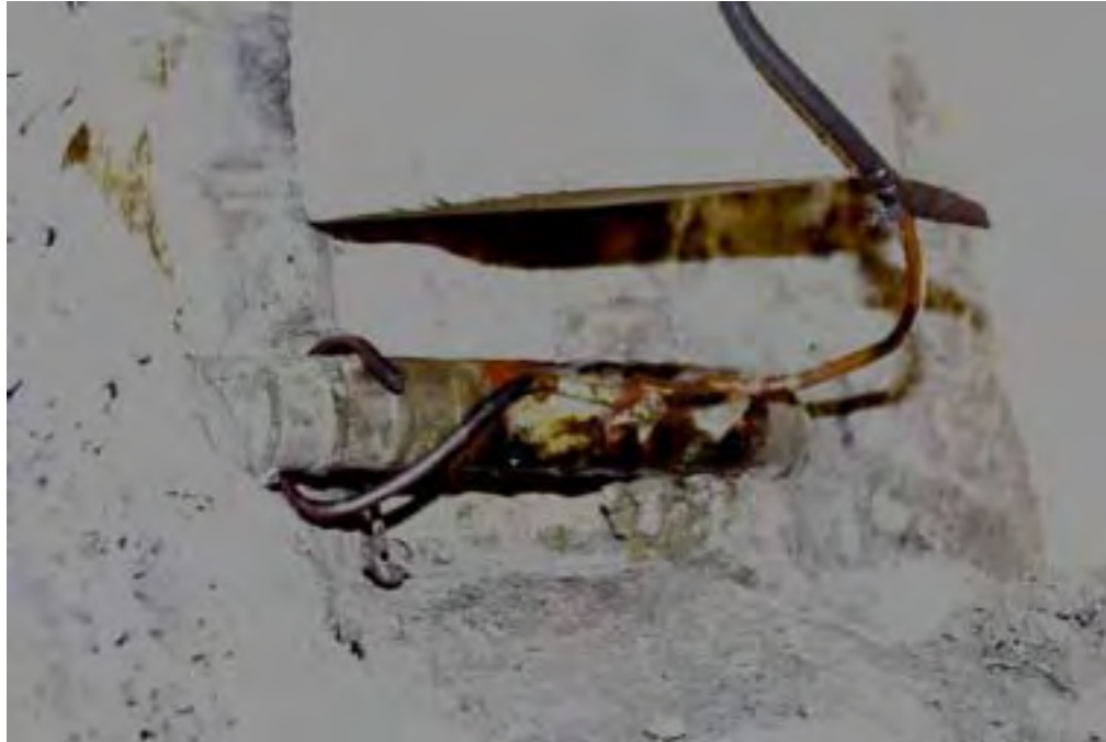
Figure 5.20 Typical silver soldered electrical connection
