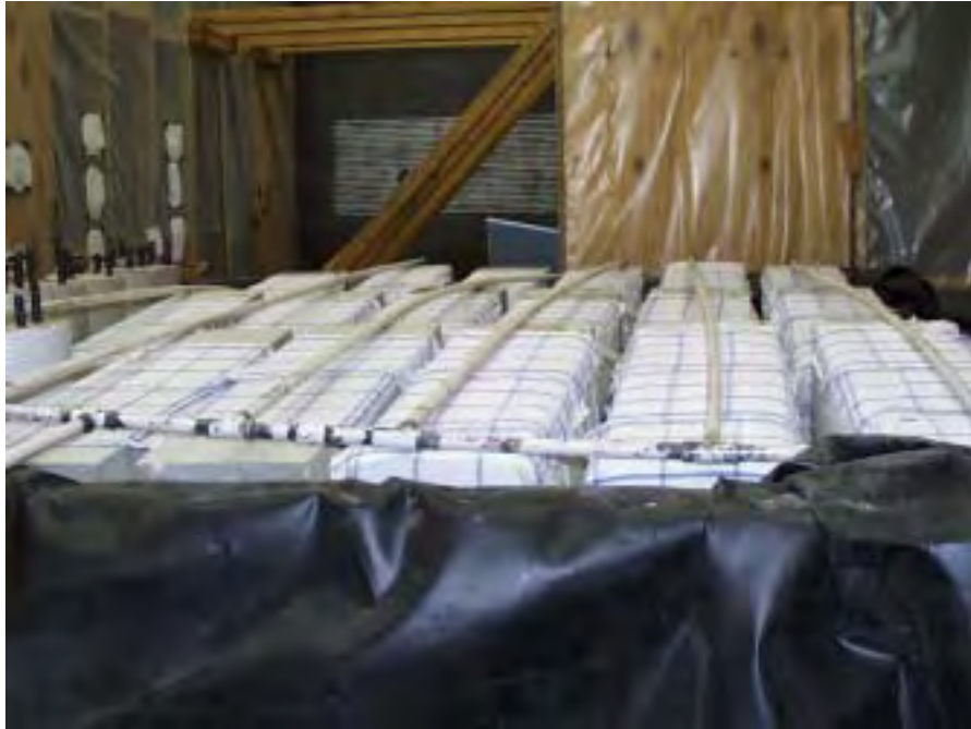
Figure 4.19 Irrigation pipes over beams
