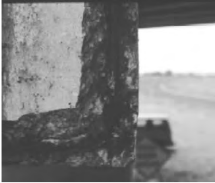
Figure 5.11 Closeup of area with severe concrete spalling
