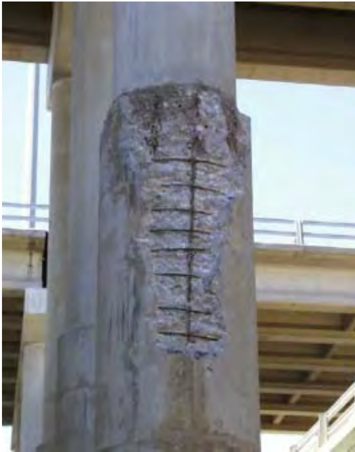
Figure 5.12 Concrete spalling on a bridge support column
