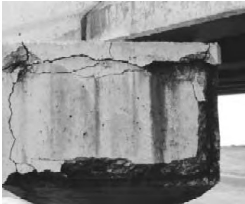
Figure 5.10 Corrosion damage on downstream endcap
