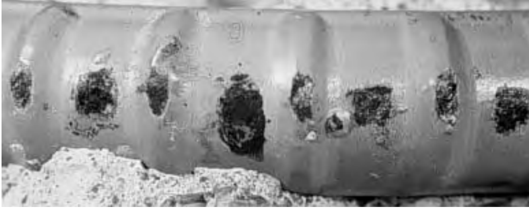
Figure 2.18 Example of 25-mm (#8) coated bar specimens after one year of exposure.
