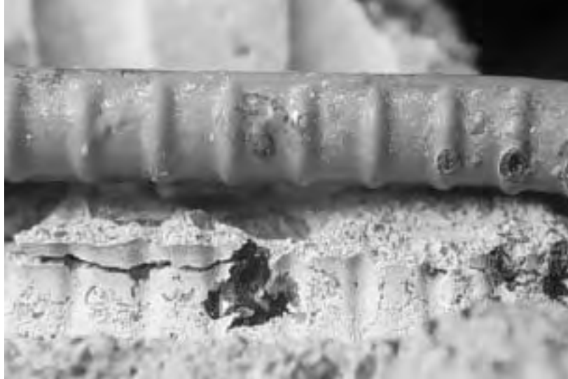
Figure 3.24 Blisters always formed adjacent to concrete voids.
