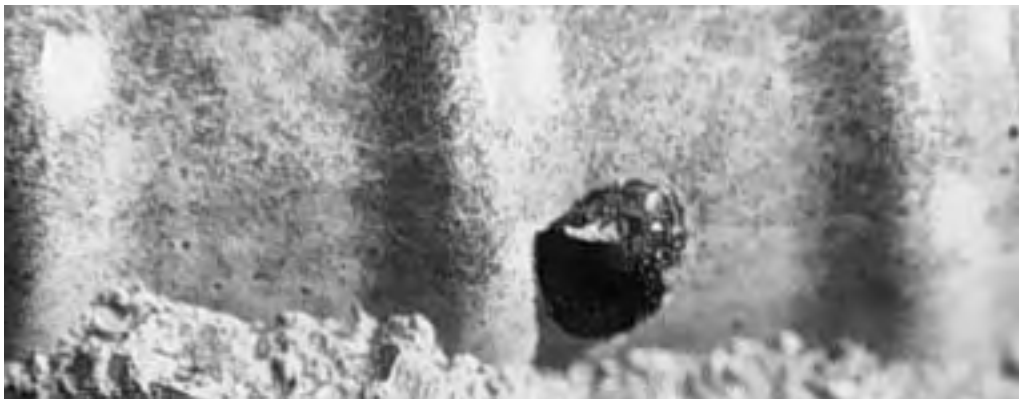
(b) Void in concrete at blister formation
