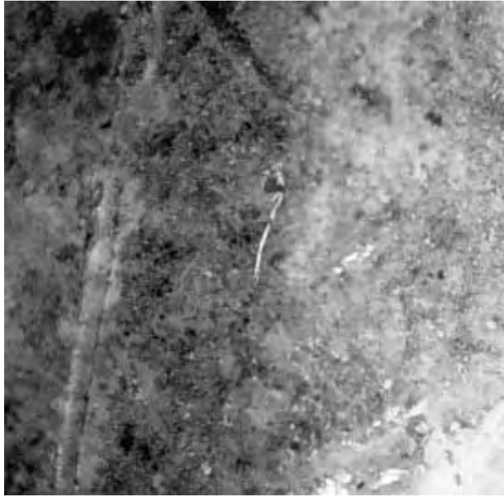
Figure 3.27 Concrete above coated bar.
