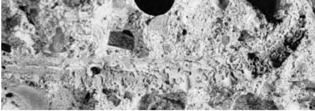
Figure 2.52 Bar trace on bottom of coated bar in concrete.
