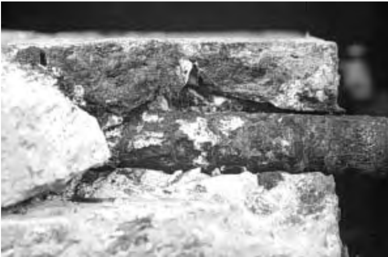
(c) Pitting at straight leg of 25-mm (#8) uncoated bar after 4.5 years of exposure.
