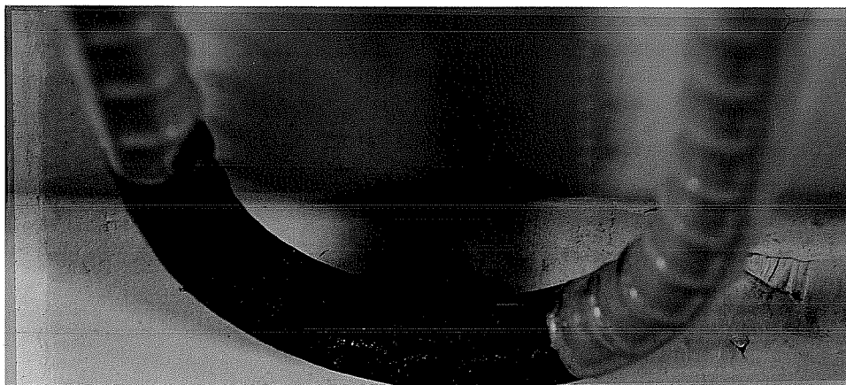
(a) The inside of bend of the bar shown in Figure 3.16(a)
