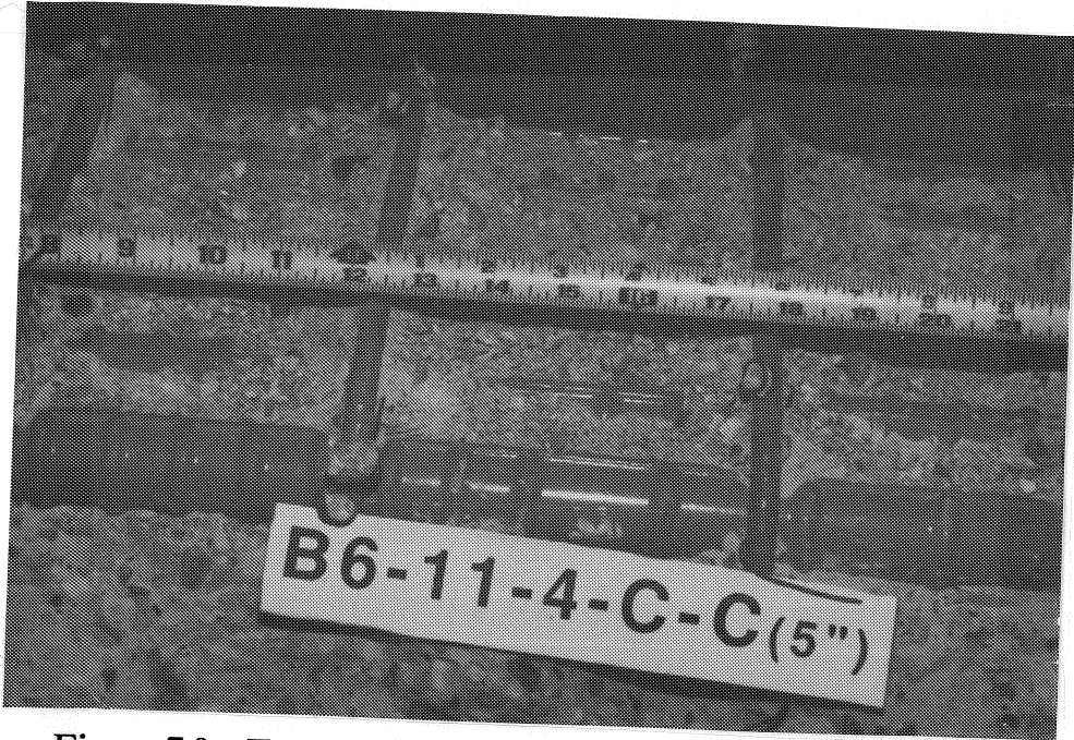
Figure 7.9 Epoxy-coated reinforcing bars after splice failure.
