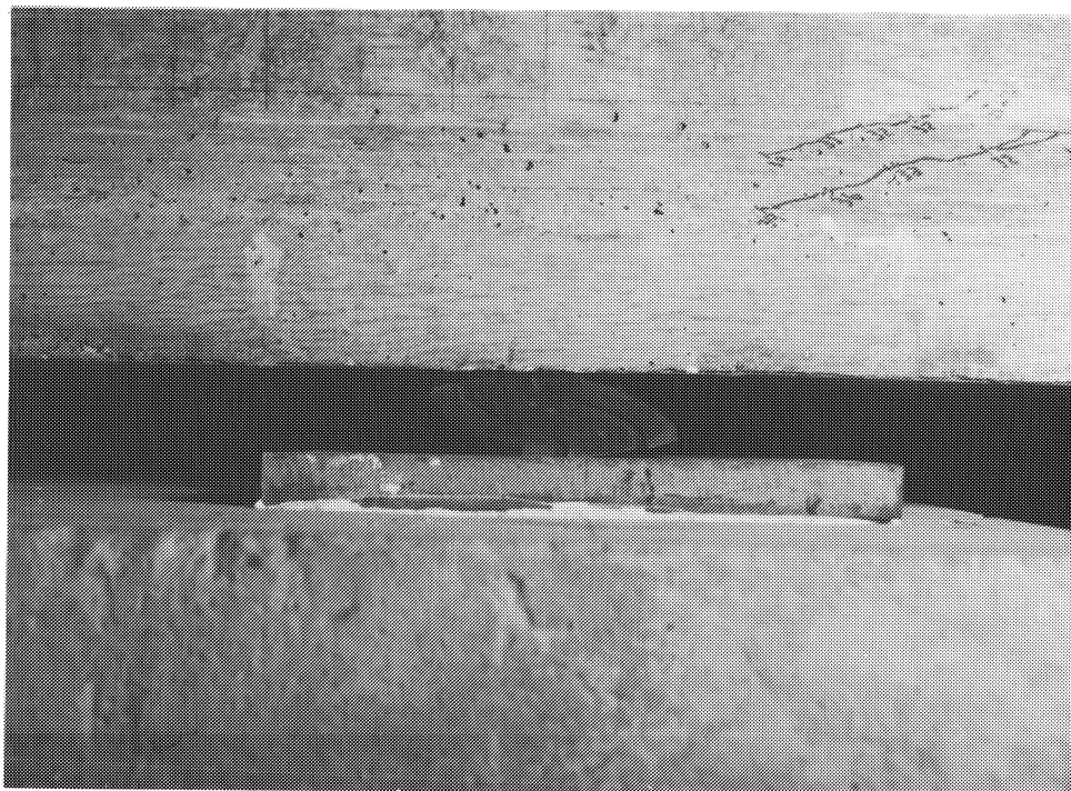
Figure 3.26 Failed elastomeric bearing during Test 1A-1-0.6.
