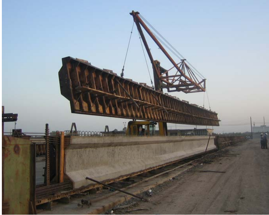
Figure 6-3: Form removal for a line of Type-IV girders at TCC Victoria plant
