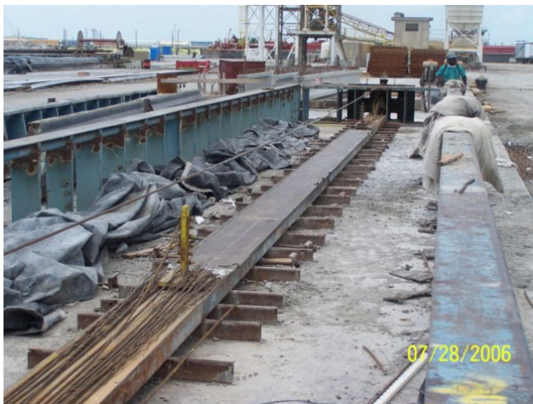
Figure 6-6: Small bed at HEI Corpus Christi plant used to cast Type-A beams (photograph courtesy of Chris Leonard)
