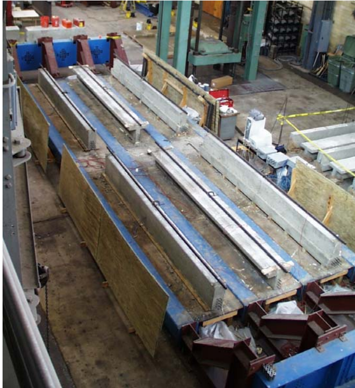
Figure 3-5: Prestressing bed with rectangular, tee, and inverted-tee beams (photograph courtesy of Alfredo Castro)
