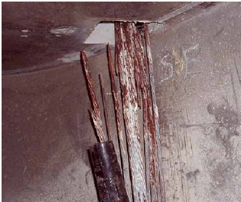
Figure 2.11 Tendon Corrosion inside the Sunshine Skyway Bridge Piers (Refer to Figure 2.3) 16
