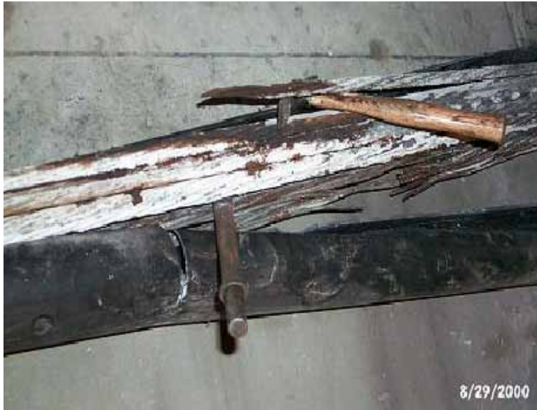
Figure 2.8 Failure of Tendon 28-6 on the Mid-Bay Bridge 16
