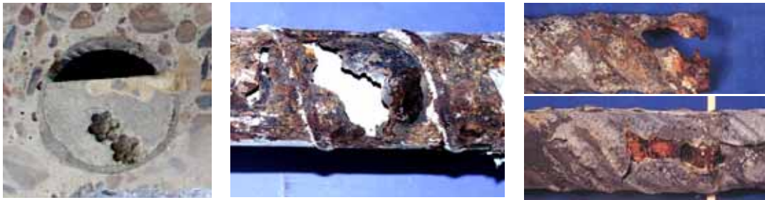
Figure 3.24 Bleed Water Voids and Duct Corrosion 37
