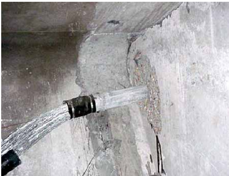
Figure 2.9 Failure of Tendon 57-1 on the Mid-Bay Bridge at Expansion Joint Diaphragm 16
