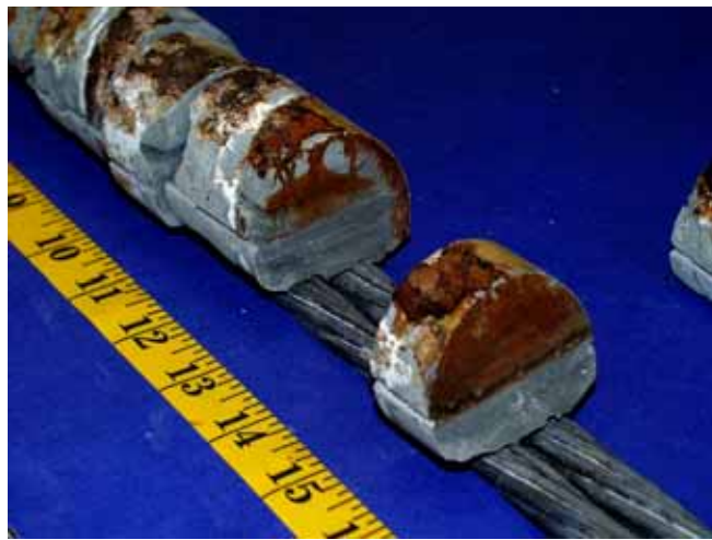
Figure 3.25 Effect of Grout Cracking 37
