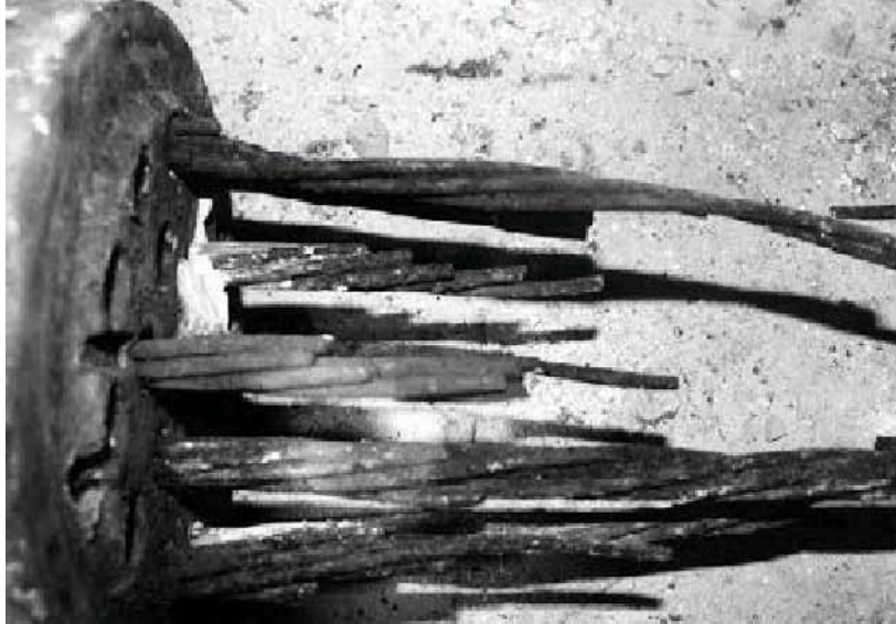
Figure 2.6 Advanced Corrosion of Strands within Anchorage Niles Channel Bridge 16
