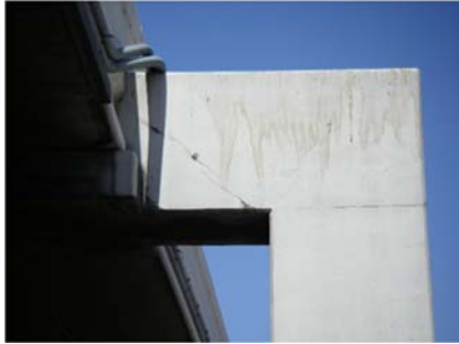
Diagonally cracked RC bent cap (Courtesy of Straddle Cracking Database OB)
